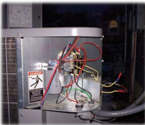
Figure 2: Traditional installation shows DCU wires (bright red, black, and blue) installed at compressor.
